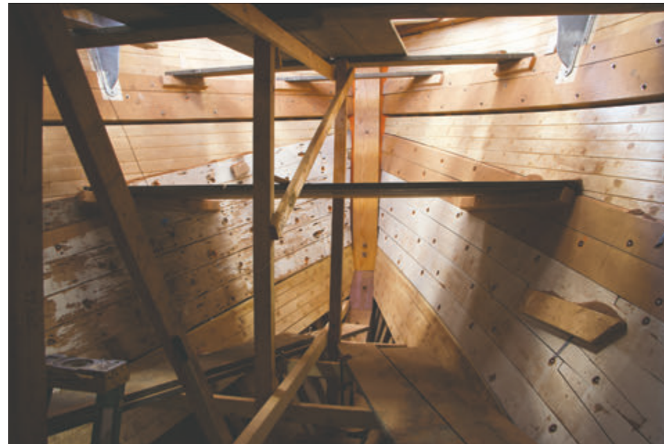
The stem of the Western Flyer as crews continue their work to restore the famed boat featured in John Steinbeck’s “The Log from the Sea of Cortez.” Leader photo by Nick Twietmeyer
