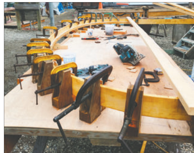
A series of clamps help hold the form of the Carlisle II's new framing for the extension to the second level passenger area top. Photo courtesy Haven Boatworks
